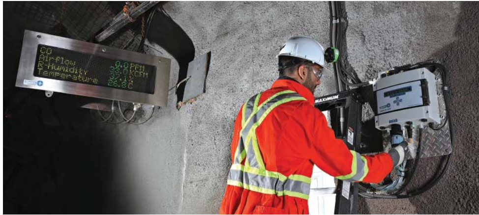
One of Maestro's air quality monitoring systems in action. (Photo: Maestro Digital Mine)
